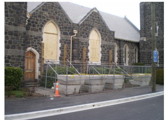
St Mary's Merivale – North Transept Wall Windows removed to safe storage and the wall supported to prevent further damage
