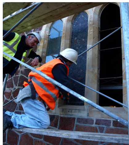
Mark Whyte of Goldfield Stone with Graham Stewart removing the historic north window at Holy Trinity Lyttelton
