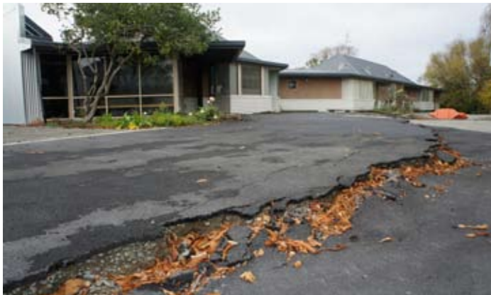
Giant cracks and major damage have meant the closure and imminent demolition of the Churchill retirement complex.
